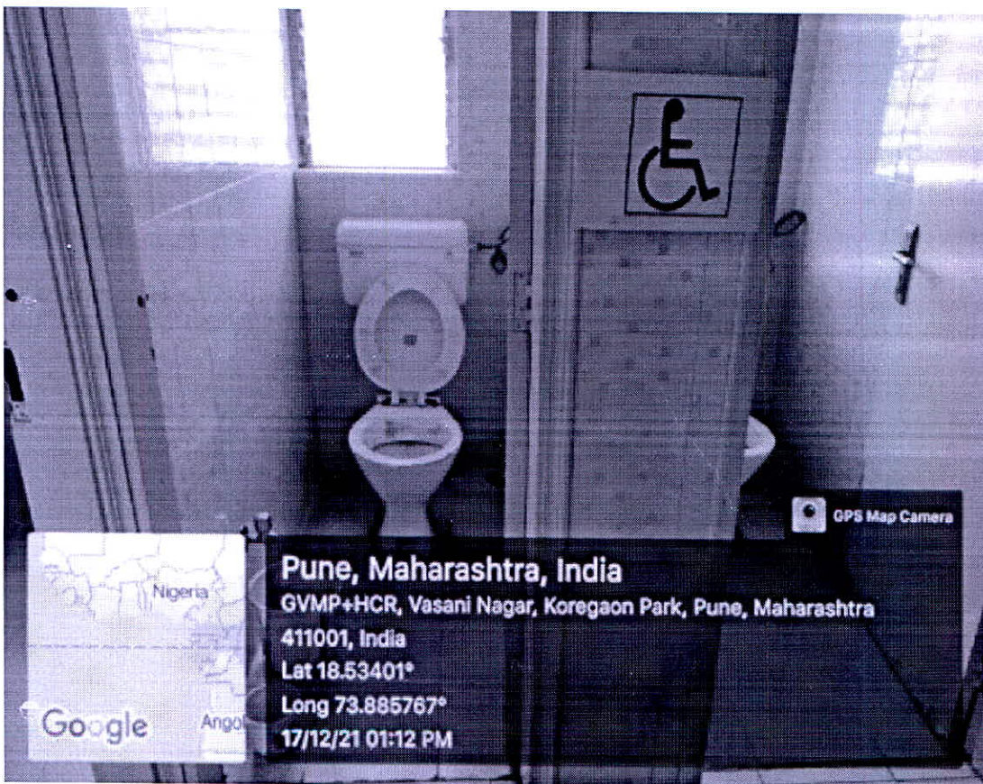
Pic 5. Washroom for specially abled
