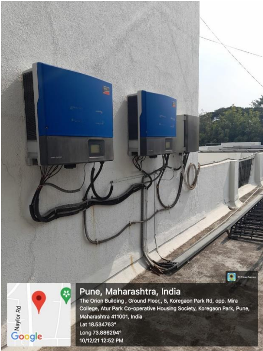
Photo 3 Solar Panel Meter
