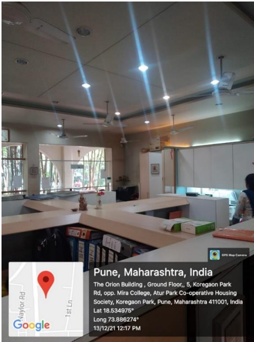
Photo 10 LED Lights - Office
