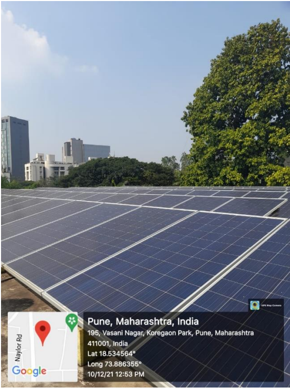
Photo 1 Solar Energy Panel
