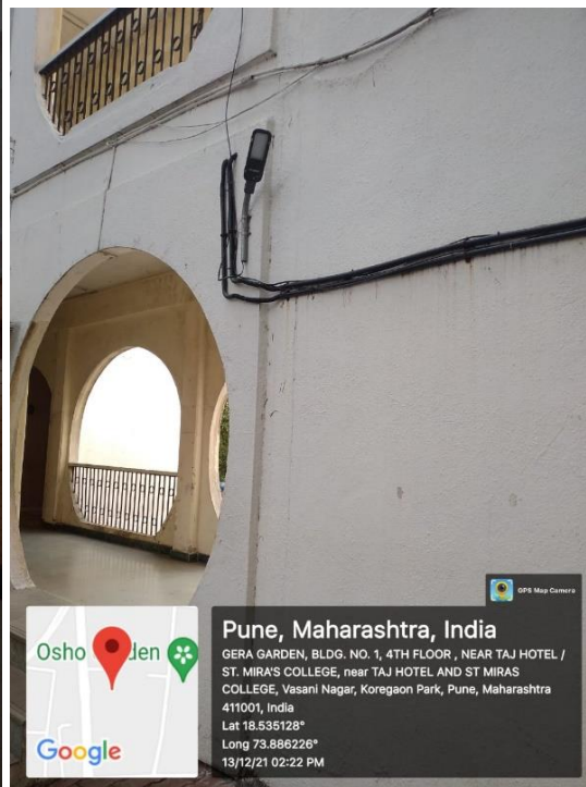
Photo 9 LED Lights – Front of Auditorium
