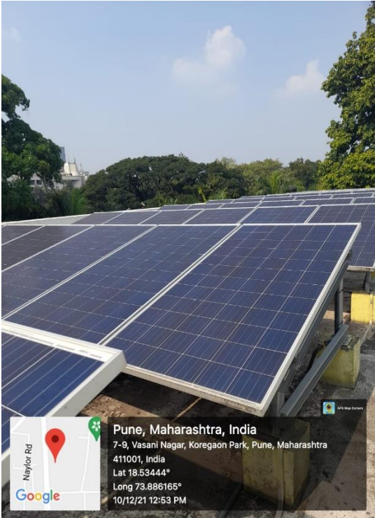
Photo 2 Solar Energy Panel
