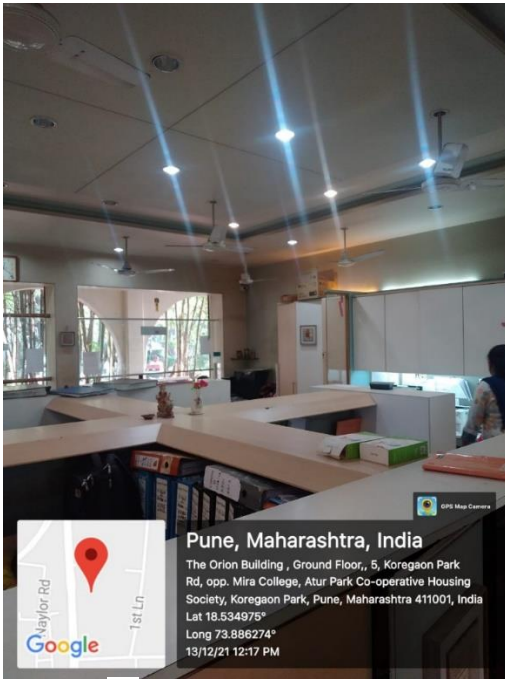
Photo 5 LED Lights - Office
