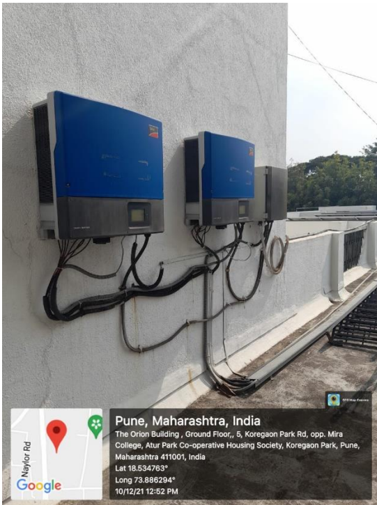
Photo 3 Solar Panel Meter
