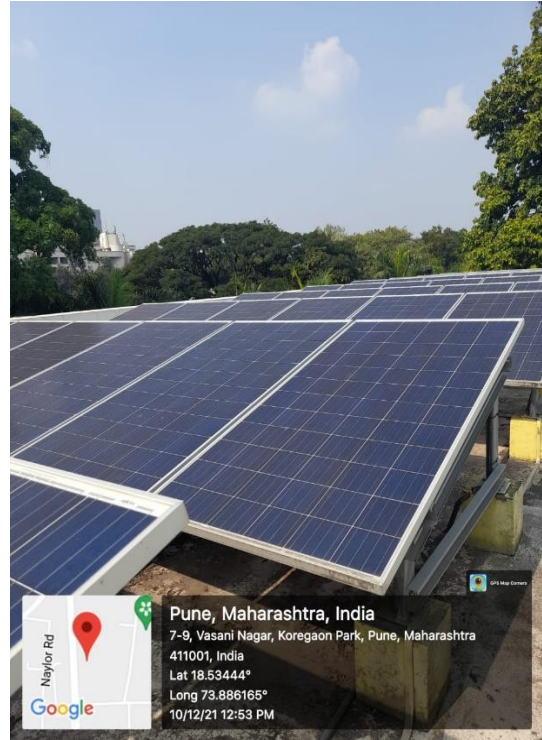
Photo 2 Solar Energy Panel
