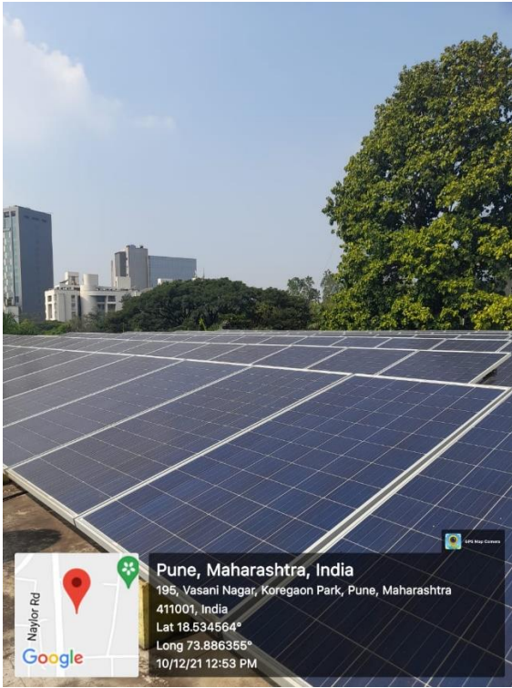
Photo 1 Solar Energy Panel
