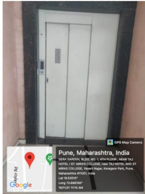
Photo 2 Lift for Specially-abled
